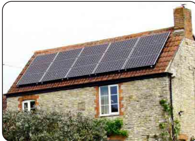
Figure 63: Example of solar panels on a roof
