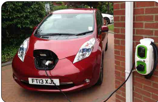
Figure 25: Off-street mounted car charging point solution
